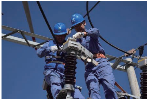
An emergency drill of Gansu Huadian Golmud Solar Power Company Limited
