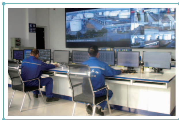
Central control room of Strong Nantong
