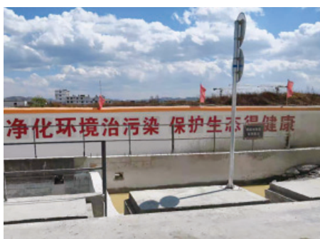
Sewage tertiary sedimentation tank 污水三級沉澱池
