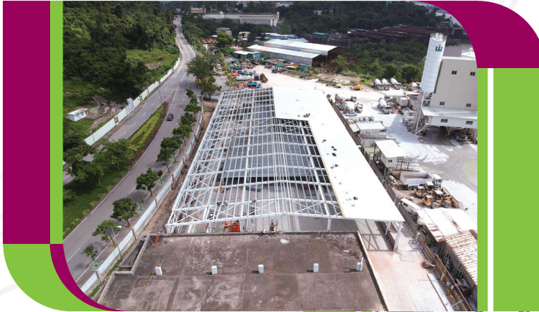
Expansion project at Lot G1, Concordia Industrial Park, Seac Pai Wan, Coloane, Macau
