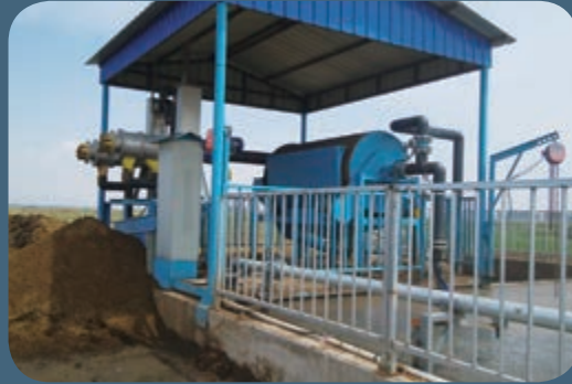
Solid-Liquid Separation System of Compost Yard
