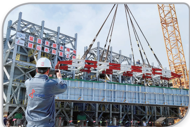
Zhejiang Petrochemical 2# ethylene plant project undertaken by the Group was awarded the title of Exemplary Civilized Construction Site
