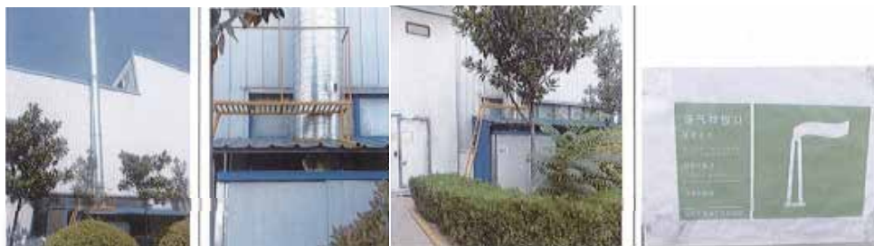
Environmental protection hosts and exhaust cylinders installed 安裝環保主機與排氣筒
