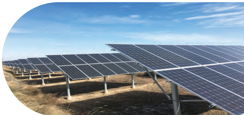
Wasion's village-level power station construction project in 2019 for photovoltaic poverty alleviation set out in the 13th Five-Year Plan
