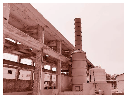
Acid mist absorption purification tower
