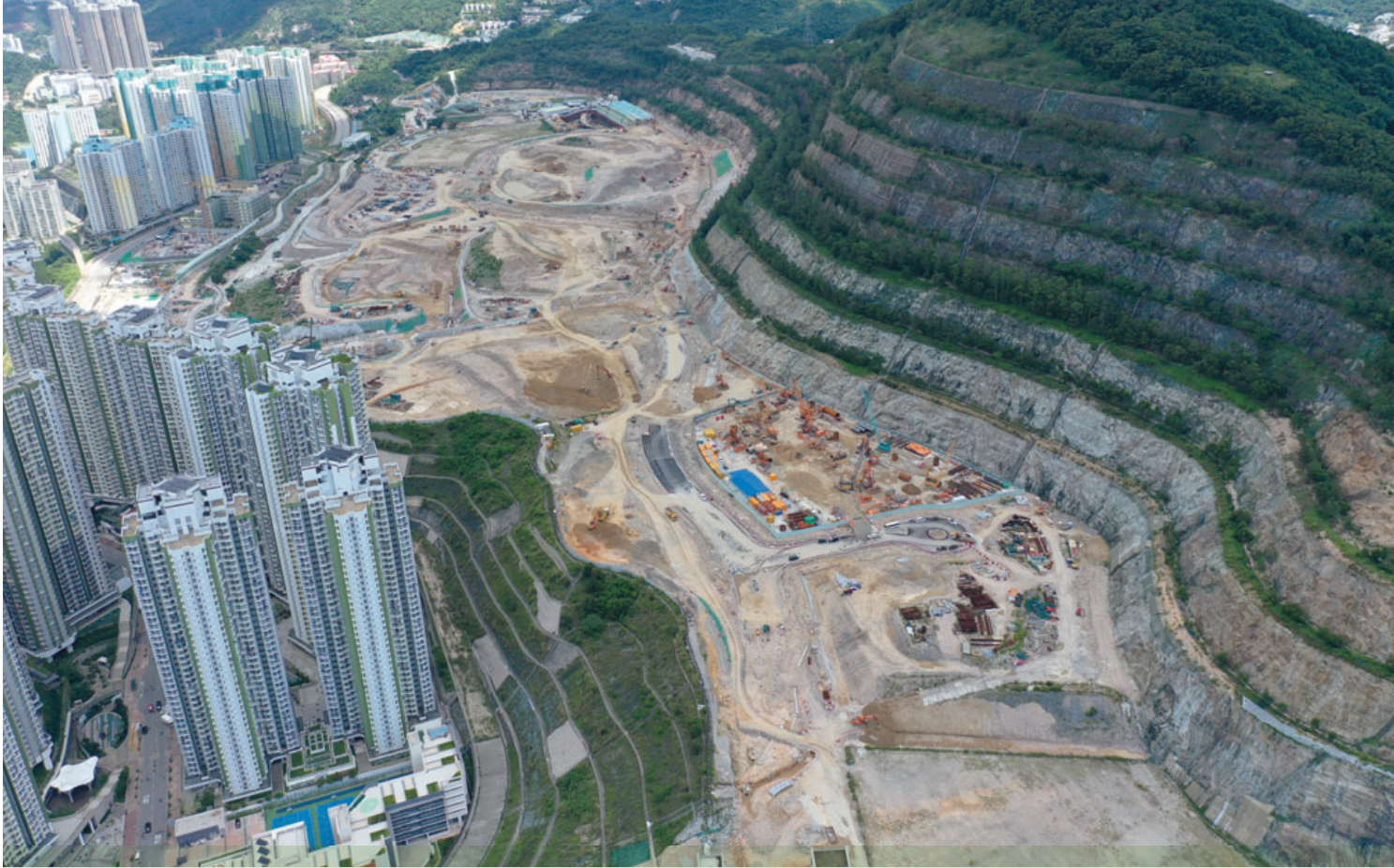
Site Formation and Infrastructure Works for Development of Anderson Road Quarry Site 安達臣道石礦場用地發展的土地平整及基礎建設工程
