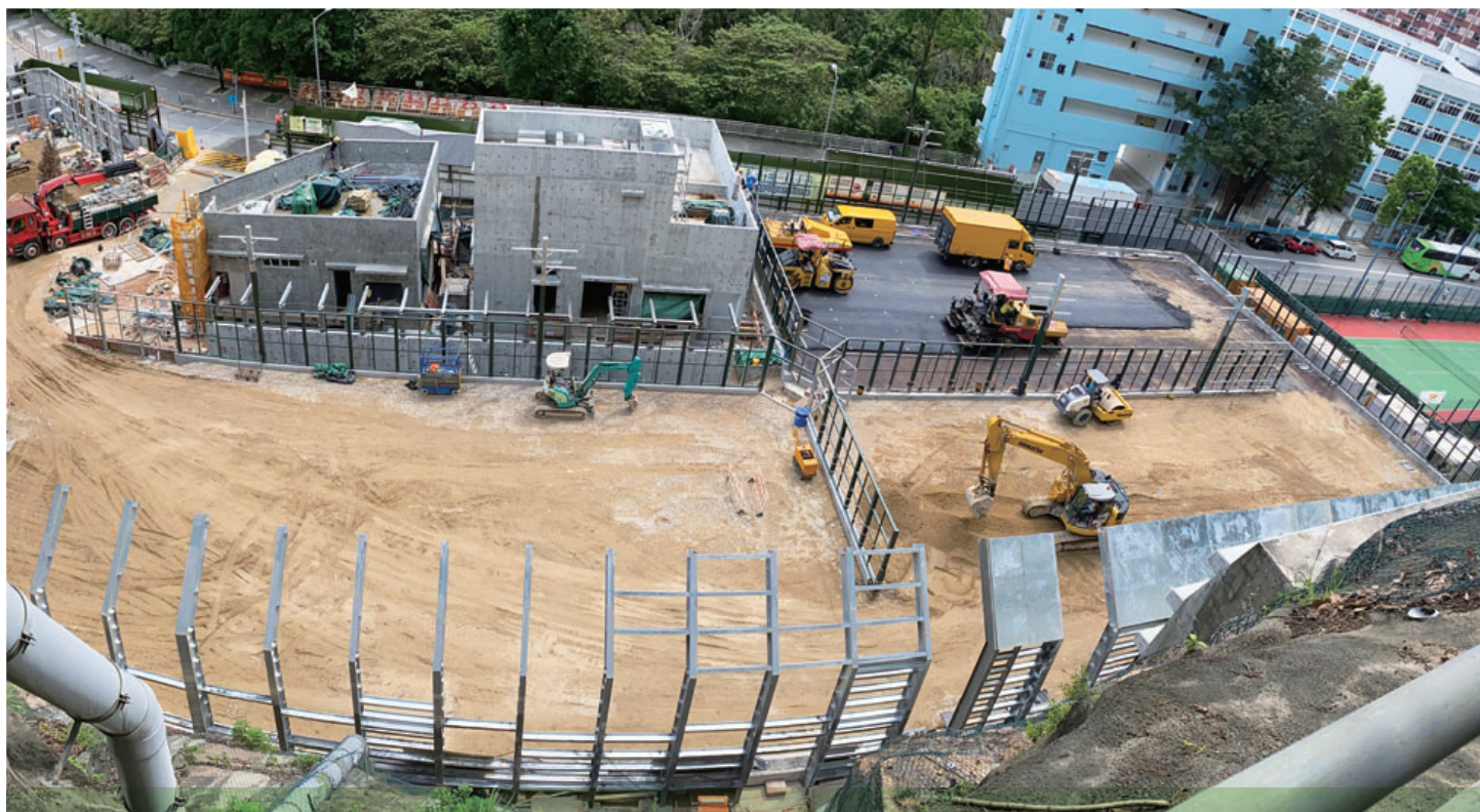
Construction of Public Housing Development at Hiu Ming Street 曉明街公營房屋發展之建造工程
