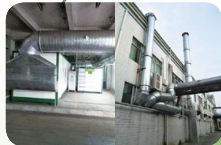
Appearance and installation of the environment-friendly VOCs treatment system VOCs環保系統外觀及配置效果圖
