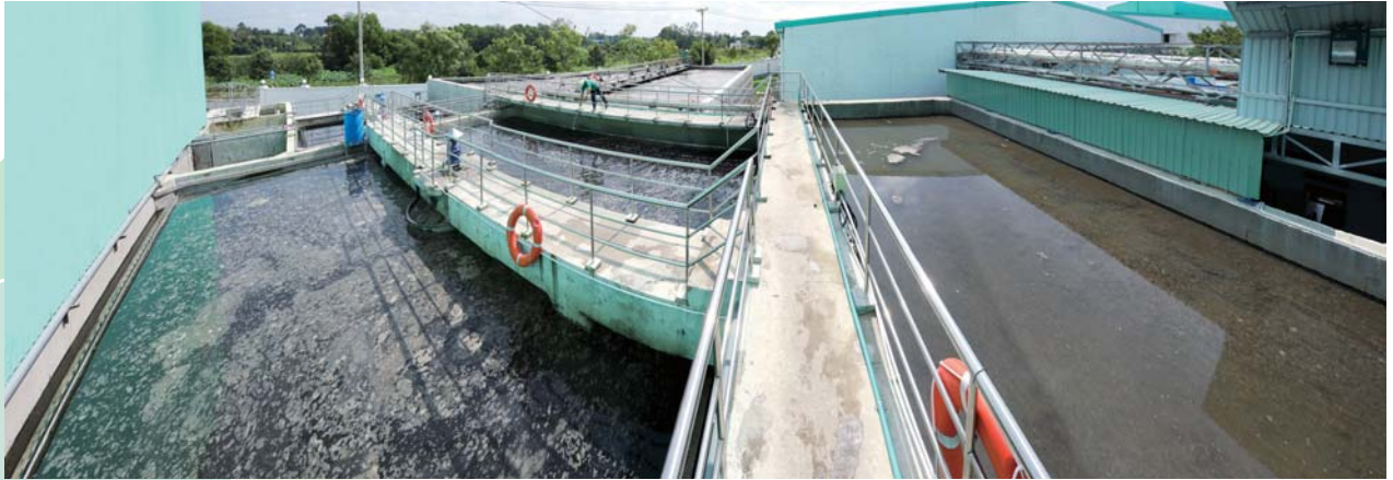
Sewage treatment facilities
