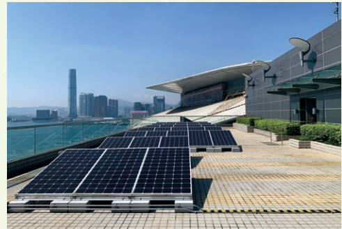
Solar panels installed at the rooftop of the HKCEC
