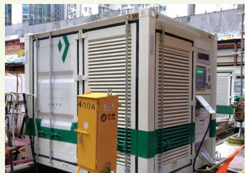
Use of "Enertainer" at construction sites
