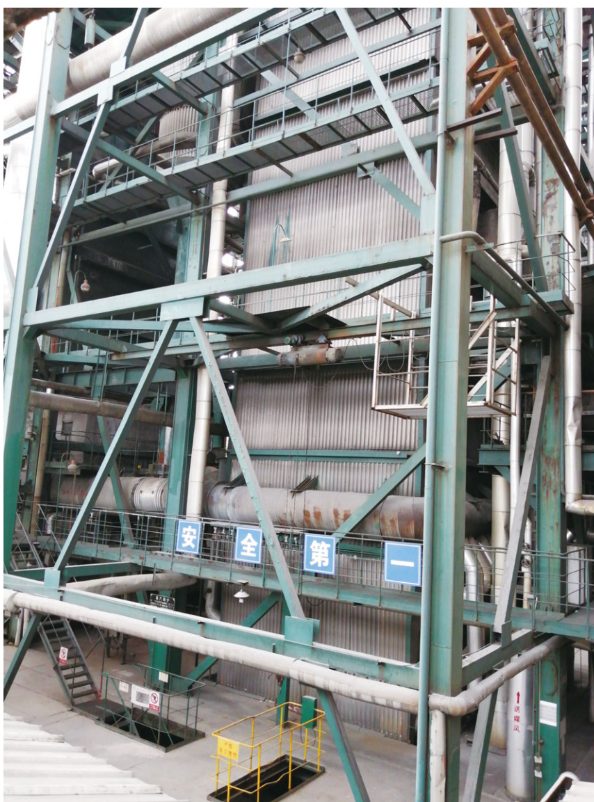
Circulating Fluidised Bed Boilers 循環流化床鍋爐
