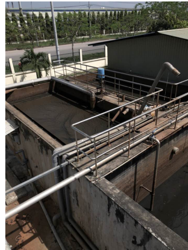
Waste water treating facilities in Dream Textile
