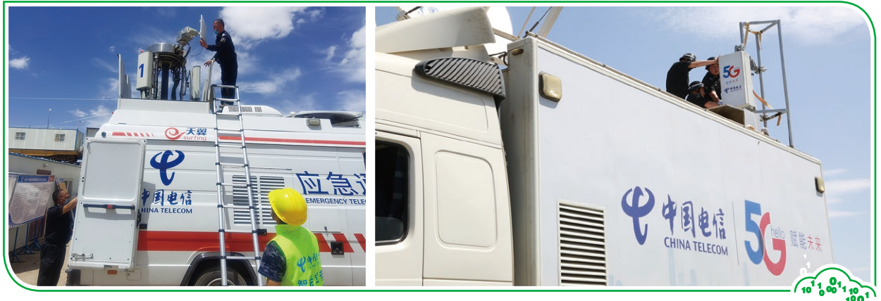
5G emergency communications assurance
