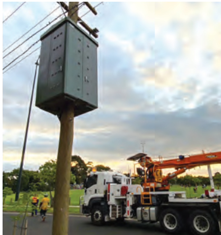
United Energy is undergoing the Bayside Battery Project, a trial involving pole mounted batteries to help manage peak demand.
