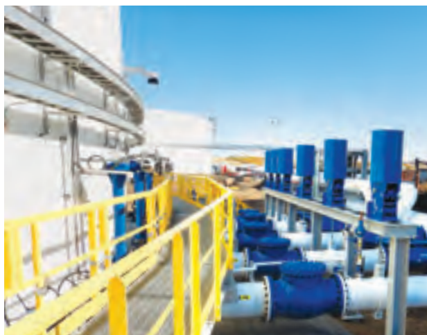
Canadian Midstream Assets expanded the crude oil storage capacity in its Hardisty terminal.
