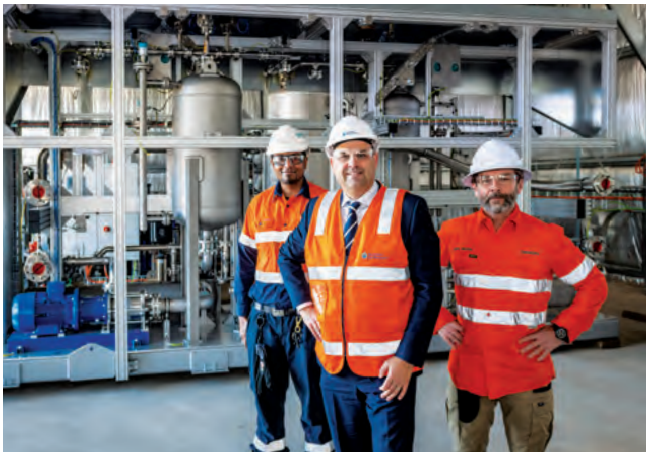
Australian Gas Networks' Hydrogen Park South Australia in Adelaide is at the final stage of commissioning. The facility will produce renewable hydrogen using a 1.25 MW electrolyser.
