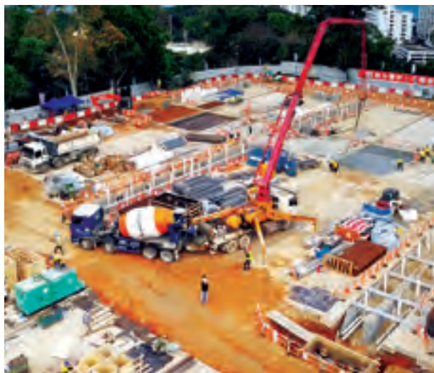
Alliance managed to maintain stable and high-quality concrete supply for the construction of two quarantine camps at Lei Yue Mun Park and Penny's Bay in the first quarter of 2020 amidst the COVID-19 outbreak.
