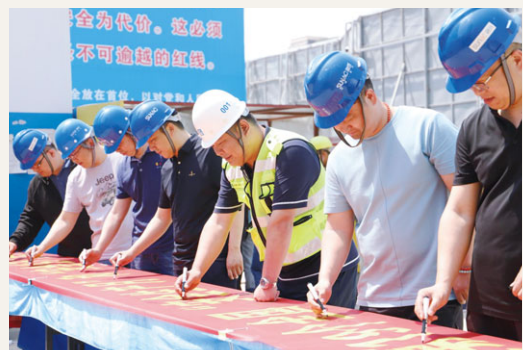
2020 Nationwide activities of "Work Safety Month (安全生產月)" – Project of Qingdao Sunac Victoria Bay Courtyards (青島融創•維多利亞灣項目)
