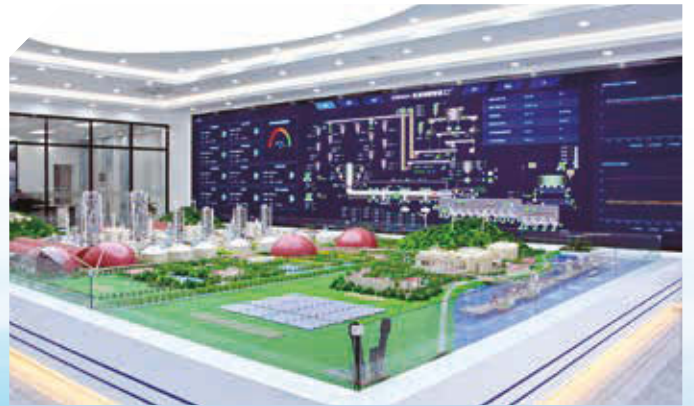
Full-process Intelligent Factory Control Room of Conch Cement
