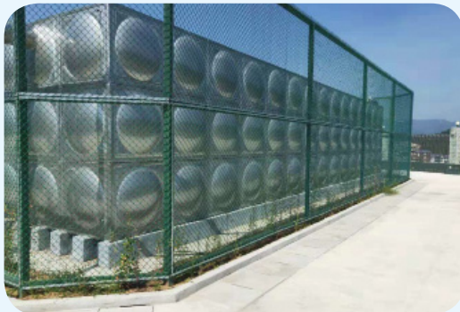
Water Supply Facility of Company B
