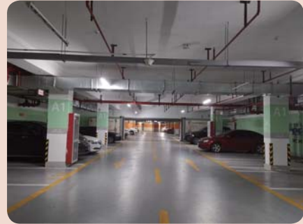
Illustration of dual-controlled LED in underground garage of Suzhou Zhongyang Tiancheng
