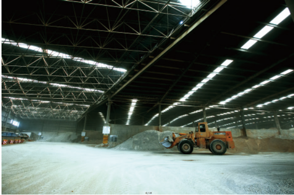
Stockyard with spraying system
