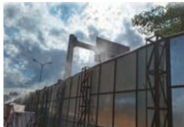
Wall block automatic spray system
