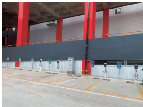
Dongguan Hongmei Park Phase II, China features EV charging facilities. It is one of three assets completed in China in 2020 for which we are awaiting the results of LEED certification.
