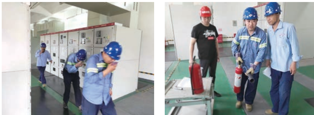
Figure: Tianbao Energy 2020 “Emergency Evacuation and Fire-fighting Exercise for Substation Fire” event
