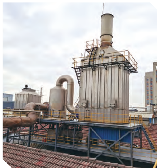
▲ Waste Gas Treatment Installation
