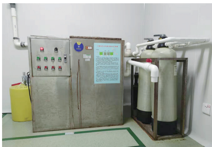
Photo: Sewage treatment equipment in Hangzhou laboratory
