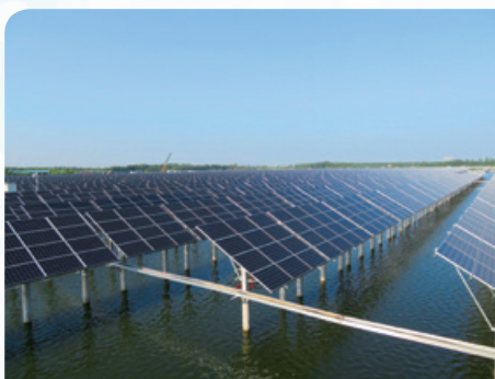
Centralised Photovoltaic Power Plant, Weishan, Shandong Province
