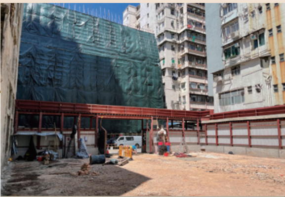
Hai Tan Street re-development project site at Sham Shui Po 深水埗海壇街重建項目地盤
