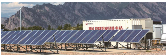
The high-performance lead-carbon battery energy storage project
