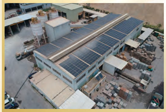
Solar panels at Hong Kong EcoPark site.
