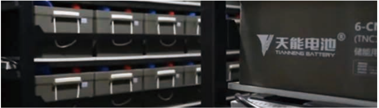
The high-performance lead-carbon battery energy storage project
