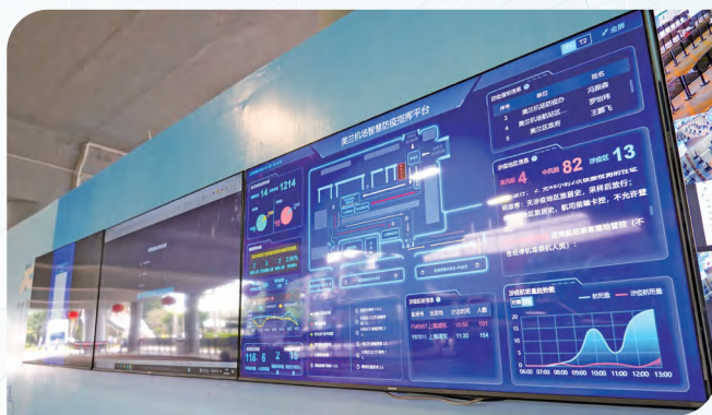
24-hour intelligent monitoring display screen 24小時智能監控顯示大屏
