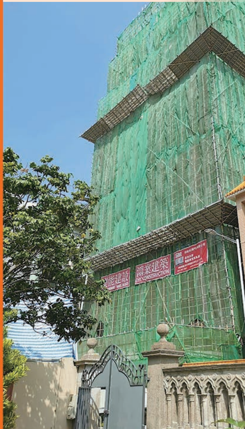
Construction works for a residential development project at Nos. 1 and 8-10 Rua de António Basto (巴士度街) and Nos. 38-40 Rua de Alves Roçadas (羅沙達街), Macau
