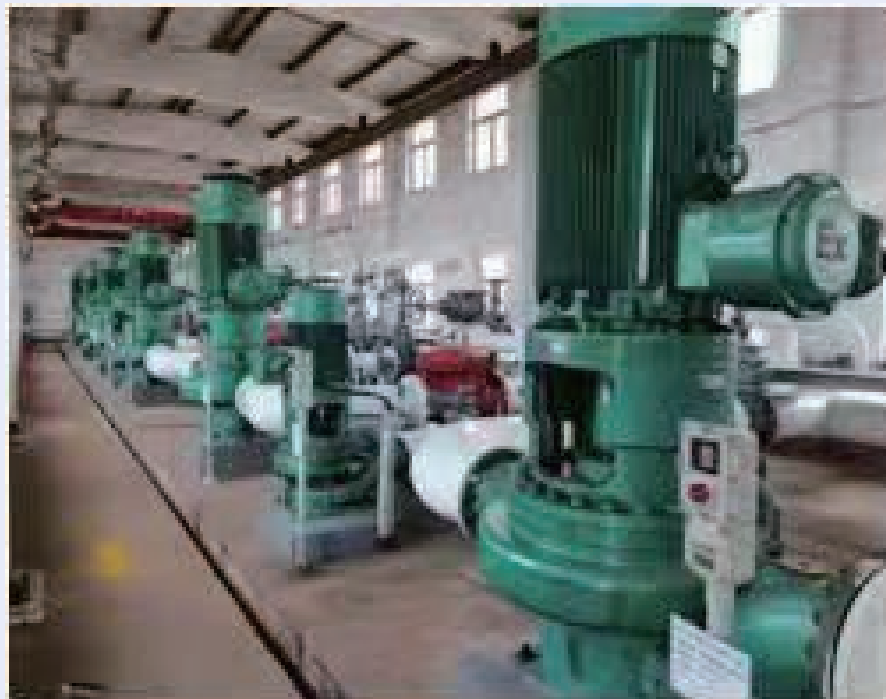
Pump temperature and vibration measurement wireless monitoring system
