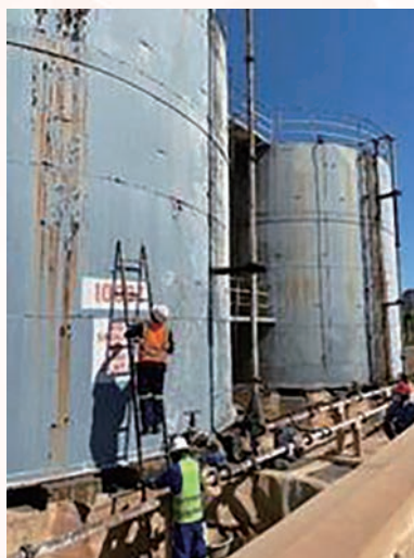
SML performs testing on specific equipment
