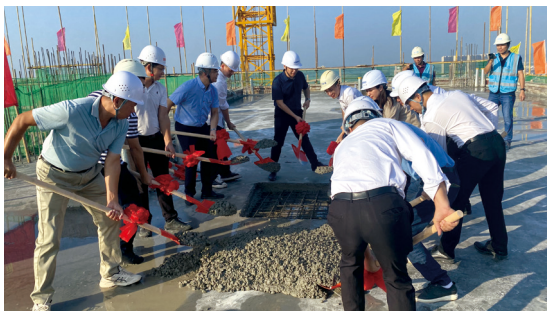
On 29 September 2021, Tower One of Chao Yang Project of the Shantou Company has its structure topped as scheduled. 於二零二一年九月二十九日，汕頭公司潮陽項目一號樓塔樓順利完成結構封頂。
