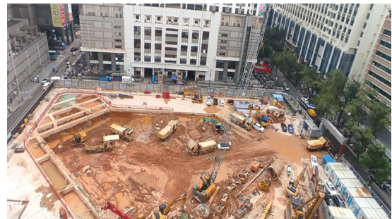
On 30 June 2021, the foundation of Shenzhen Baoxin Mansion was laid down as scheduled. 於二零二一年六月三十日，深圳寶新大廈項目樁基施工順利完成。
