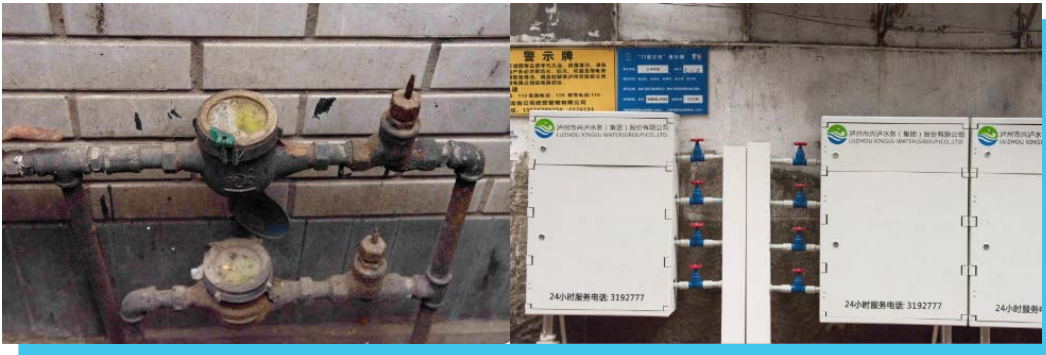
Photos of the master meter before the renovation
