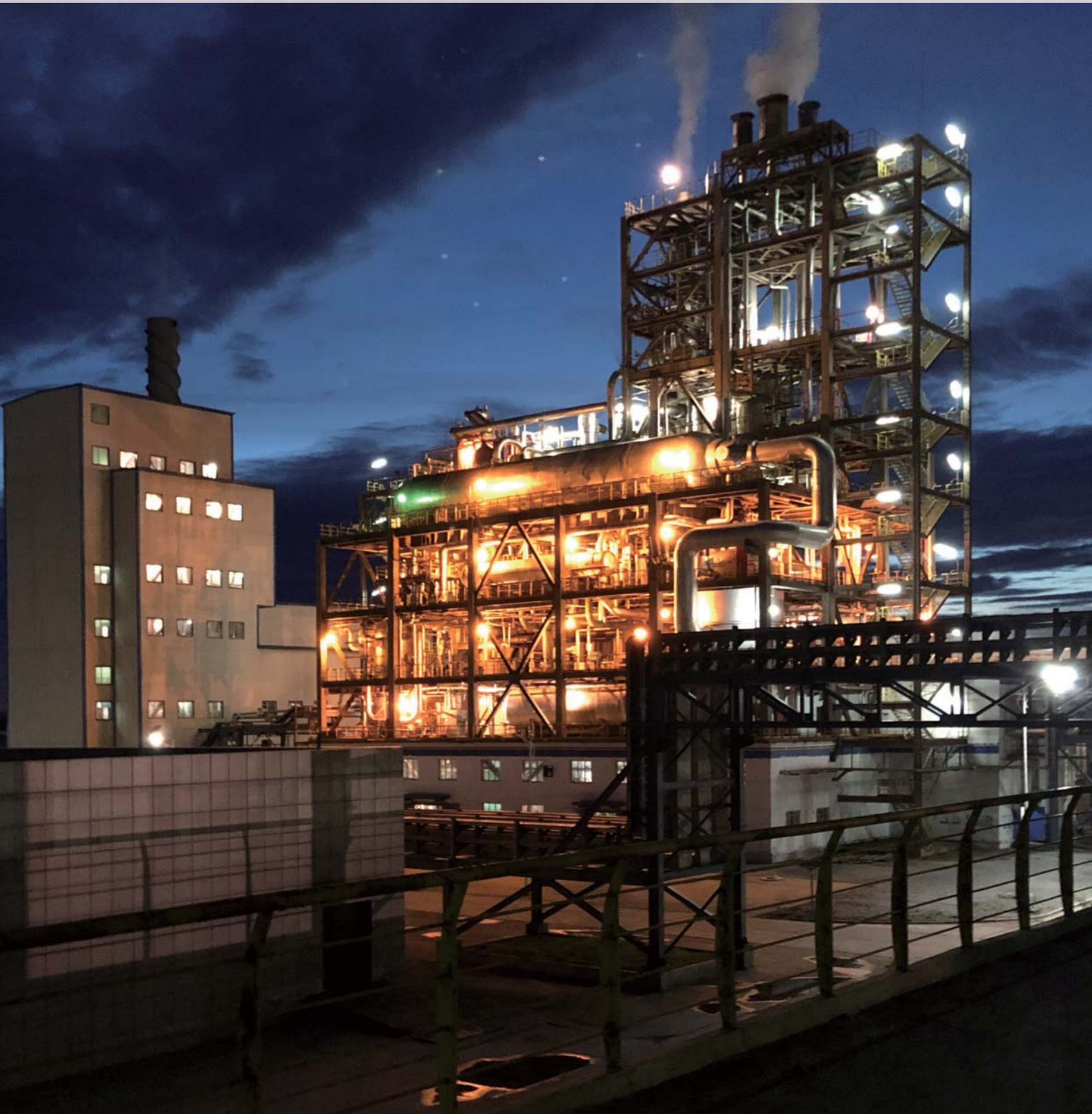
▼ CNOOC Huahe urea plant
