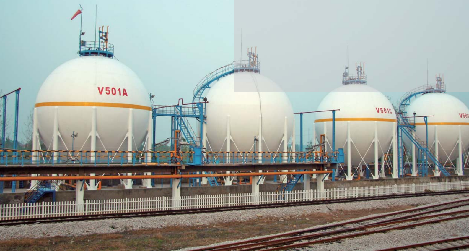
▲ DYK Chemical liquid ammonia tank
