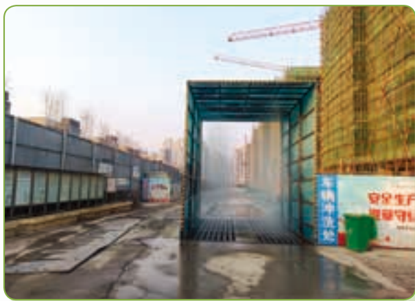
Vehicle washing facility
