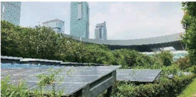
Renewable energy transformation engineering for the projects' garages
