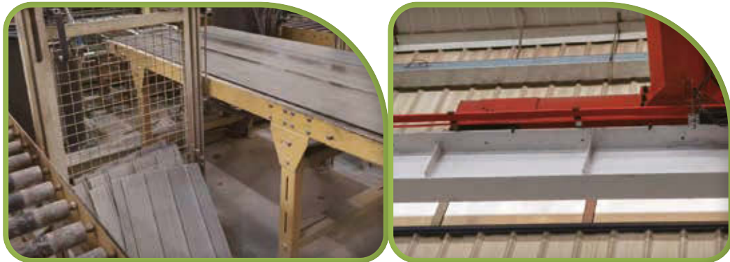
Equipment safety shield cover and overhead crane grounding wire protection measure
