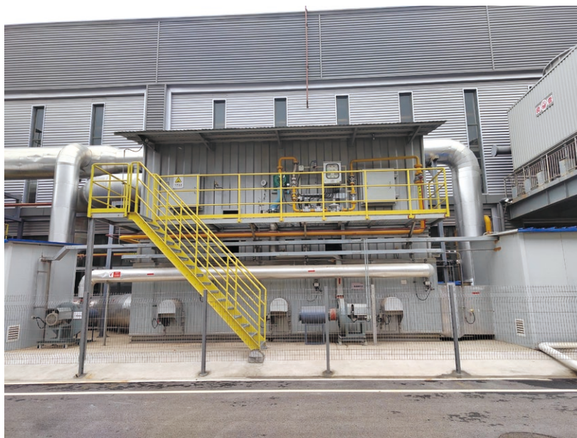
RTO treatment equipment in the Anhui production base
