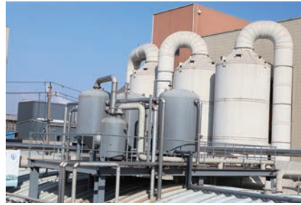
Anaerobic tower of sewage station
