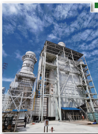
Waste heat boiler
