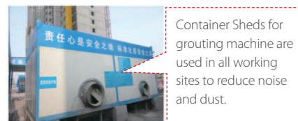
Container Shed for Grouting Machine
