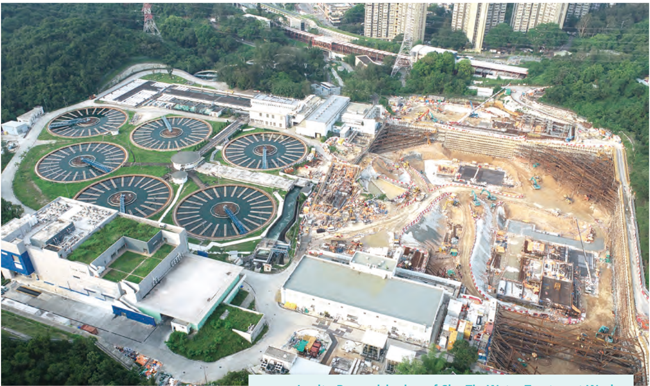
In-situ Reprovisioning of Sha Tin Water Treatment Works (South Works) – Water Treatment Works and Ancillary Facilities 沙田濾水廠原地重置工程（南廠）－濾水廠及附屬設施
