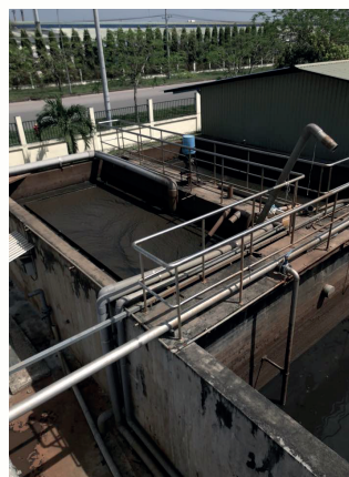
Wastewater treating facilities in Dream Textile
