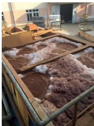
Micro-organism treatment of domestic wastewater in J.Y. Plasteel
