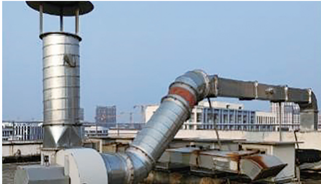
Waste gas treatment facility 廢氣處理設施
