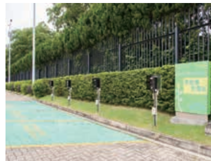
Electric vehicle charging areas
